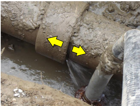
Figure III - Tension effects in AC pipe joint, Sewell Street Kaiapoi, axially aligned with the Darfield epicenter, 2010
