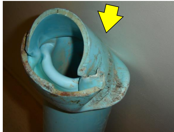
Figure XII - Ductile axial compression folding in PVC-U pipe, Gayhurst Road overbridge
