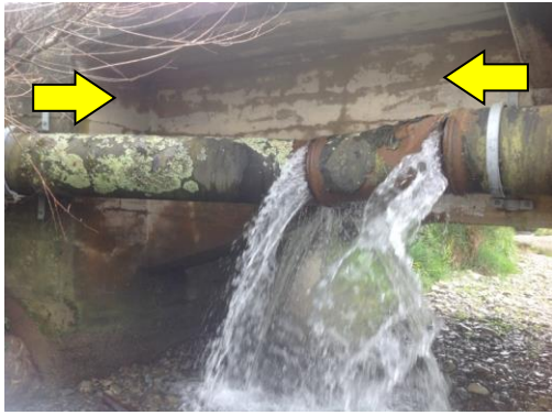
Figure V - Compression distortion and separation of RRJ joints in CLS watermain, 2014
