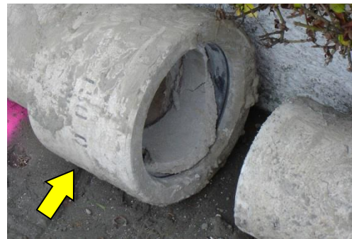
Figure VIII – Shear effects in AC pipe joint, Jollie Street, Kaiapoi, with tangential alignment to the Darfield epicenter, 2010
