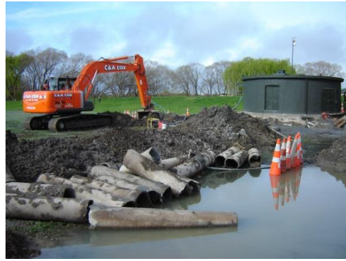
Figure VI – Compression fractures of pipe ends and joints in AC sewer rising main, Charles St, Kaiapoi, axially aligned with the Darfield epicentre, 2010 (Replaced with Biaxially Orientated PVC (PVC-O)
