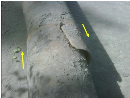
Figure IX - Compressed joint movement in CLS water main, Christchurch
