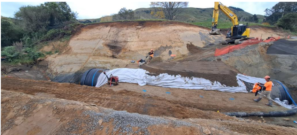
This lucky DN3200 is now protecting the people of Patoka near SH5 upstream from Eskdale
